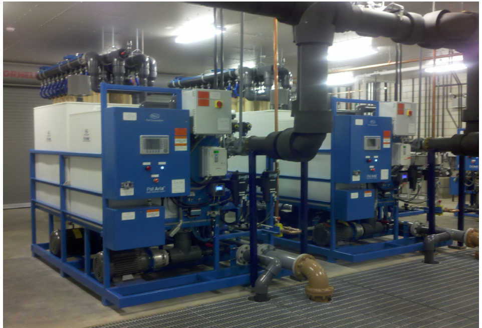
One of two 350 GPM microfiltration systems in the plant referenced in the article.
